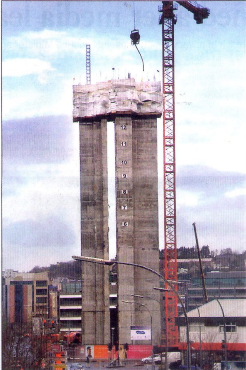
The lift shaft of the Elysian Tower has been growing at a rate of roughly one floor per day, but while the building will be Ireland's tallest when it is built, that title may only last until the development of the Dublin docklands.
